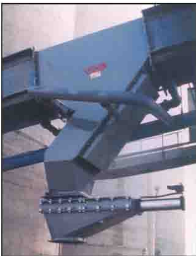
Aerated lump trap with slide gate valve.
