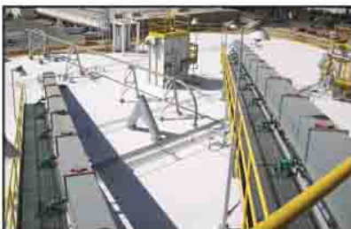
Aeration conveyors feeding multiple silos.
