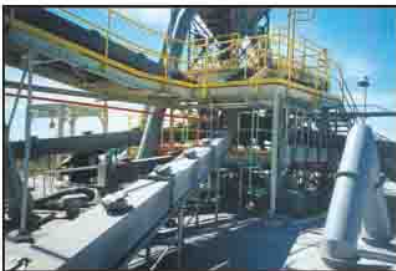
Aeration conveyor run.
