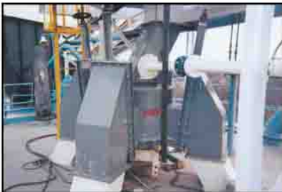
Aerated distribution box with four discharges.
