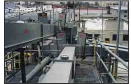
Aeration conveyors distributing to multiple silos using a combination of turning boxes and vertical slide gates.
